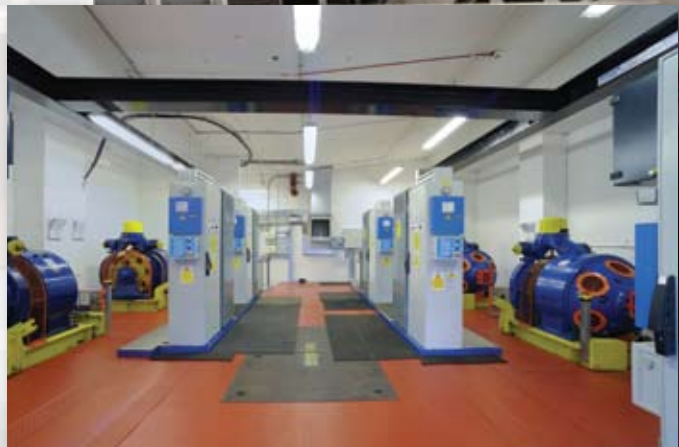
Apollo House Motor Room
